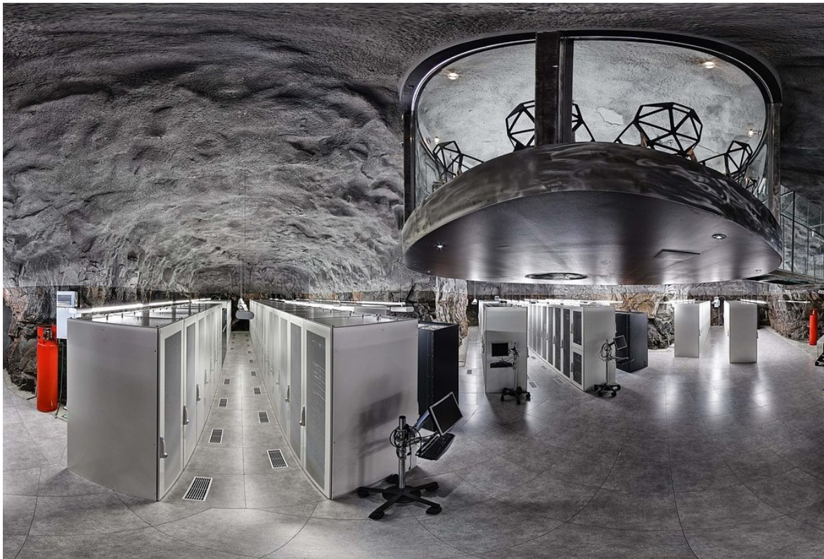
Fig. 7.1: Data centre and office building of the Swedish internet-providing company Bahnhof AB (UGE, 2020)
