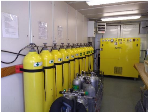
Fig. 2. Compressor van with heating system top left.
