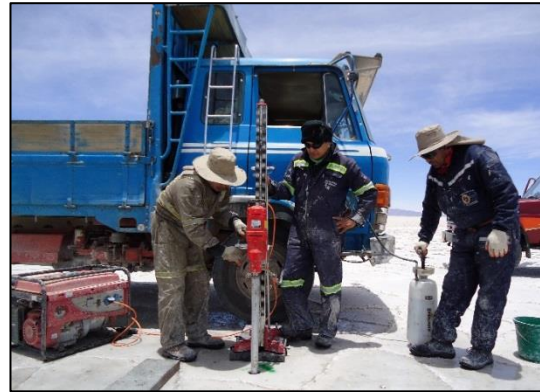
Fig. 13: Core drilling with a hand drill using the pore brine as drilling fluid
