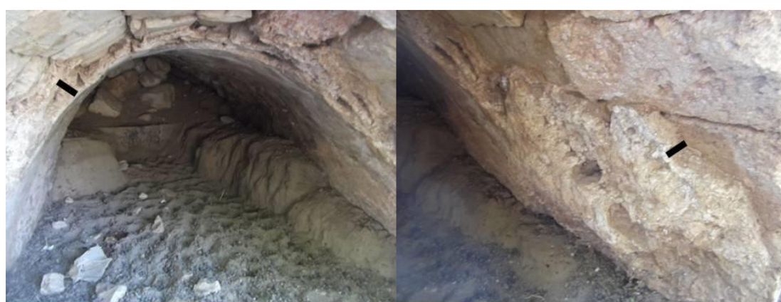
Figure 100: Water outlet at the watermill at Al Malih, shows the accumulation of the carbonate (Photo taken by Raghid Sabri 2011)
