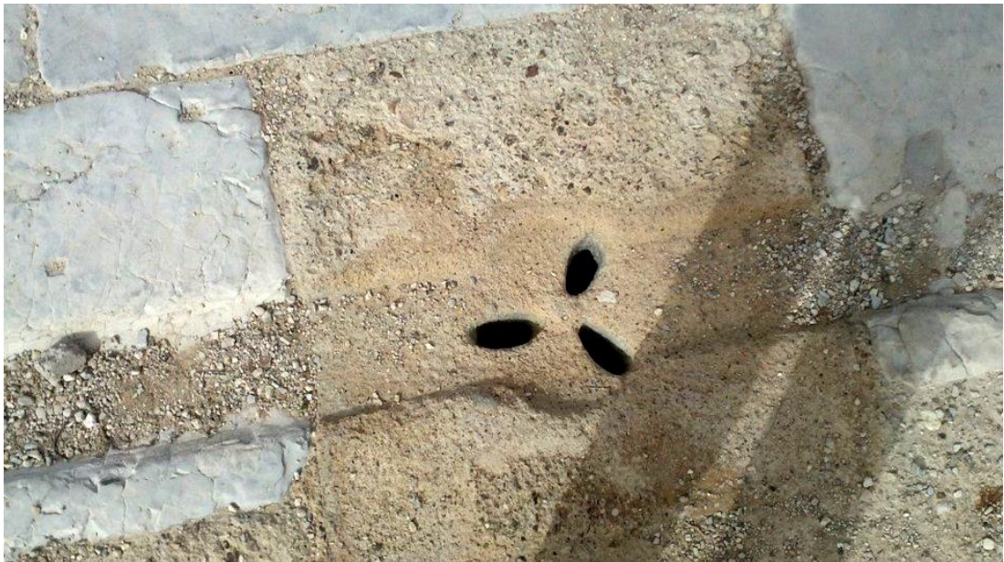
Figure 10: Rainfall drain at Hisham Palace that was utilized until the 1400 A.D. (Whitcomb 1988) (Photo taken by Nidal Zorba)
