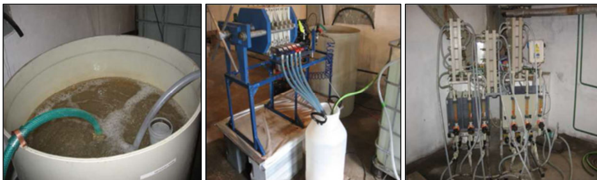
Fig. 5: Pilot aeration tank (left), filter press (center) and electro dialysis (right)
