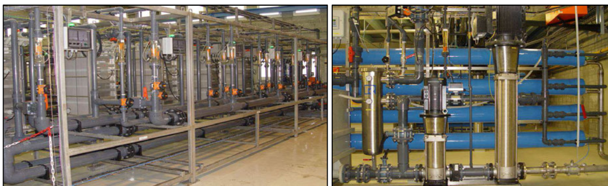
Fig. 3: Industrial electro dialysis and reverse osmosis in GEAM plant (Toman 2009)
