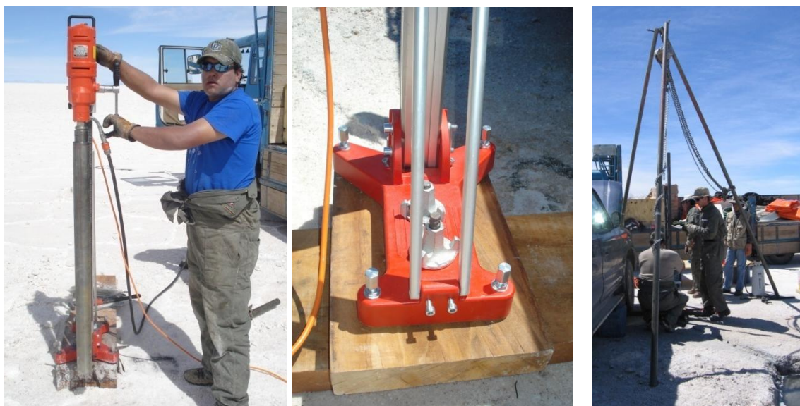
Fig. 8: Diamasa drilling machine (left); fixation of the drill rig with anchors (middle); using the support of the tripod (right)
