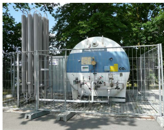
Fig. 2: Tank of liquid CO 2 (provided by company Linde), Heat exchanger. The gas has been transported gaseous from the shore to the platform (pressure 8 – 9 bar).
